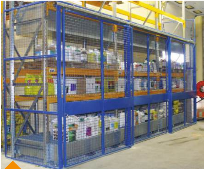
Partitioning with sliding doors to limit access to chemicals stored on heavy-duty racking on drip trays.
